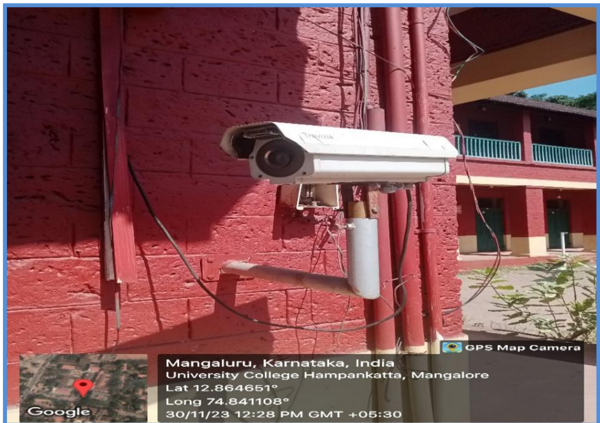
Closed - Circuit Camera positioned within the Commerce Block
